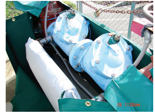
Open for servicing
